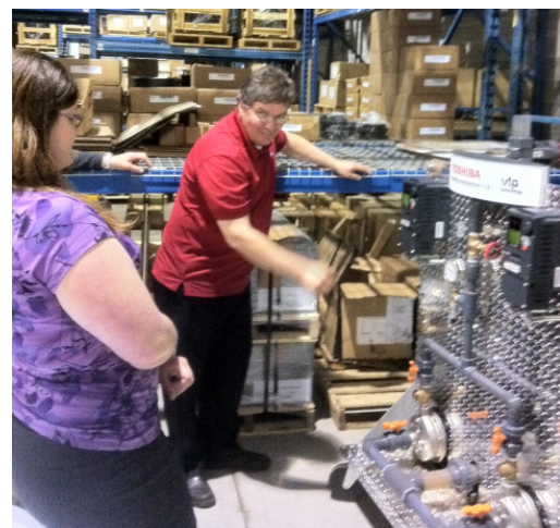
ISA Hamilton member Andrea Loar looks on as Chris Rowles from Toshont shows how multiple VFDs can be used to do automatic load-sharing in pumping applications.
